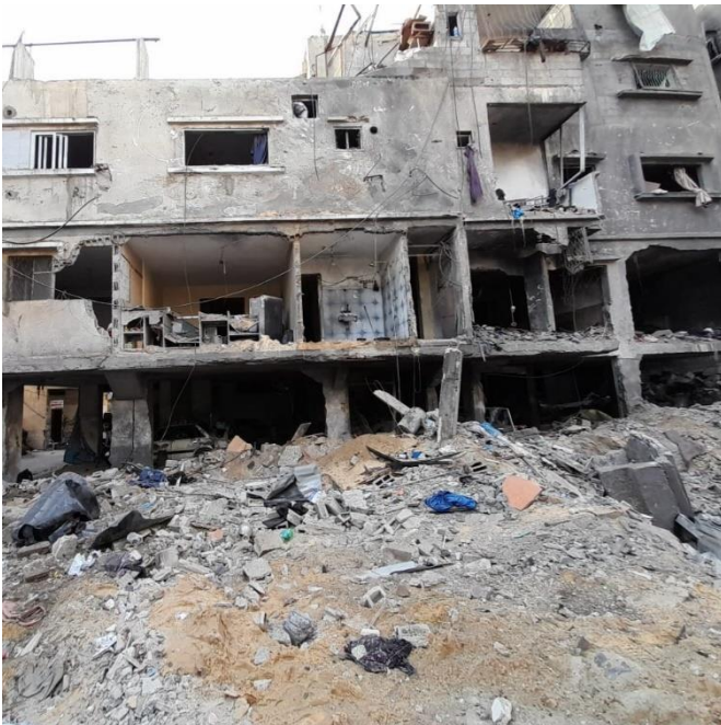
Damage caused to the Abu Mu'eileq family home.
