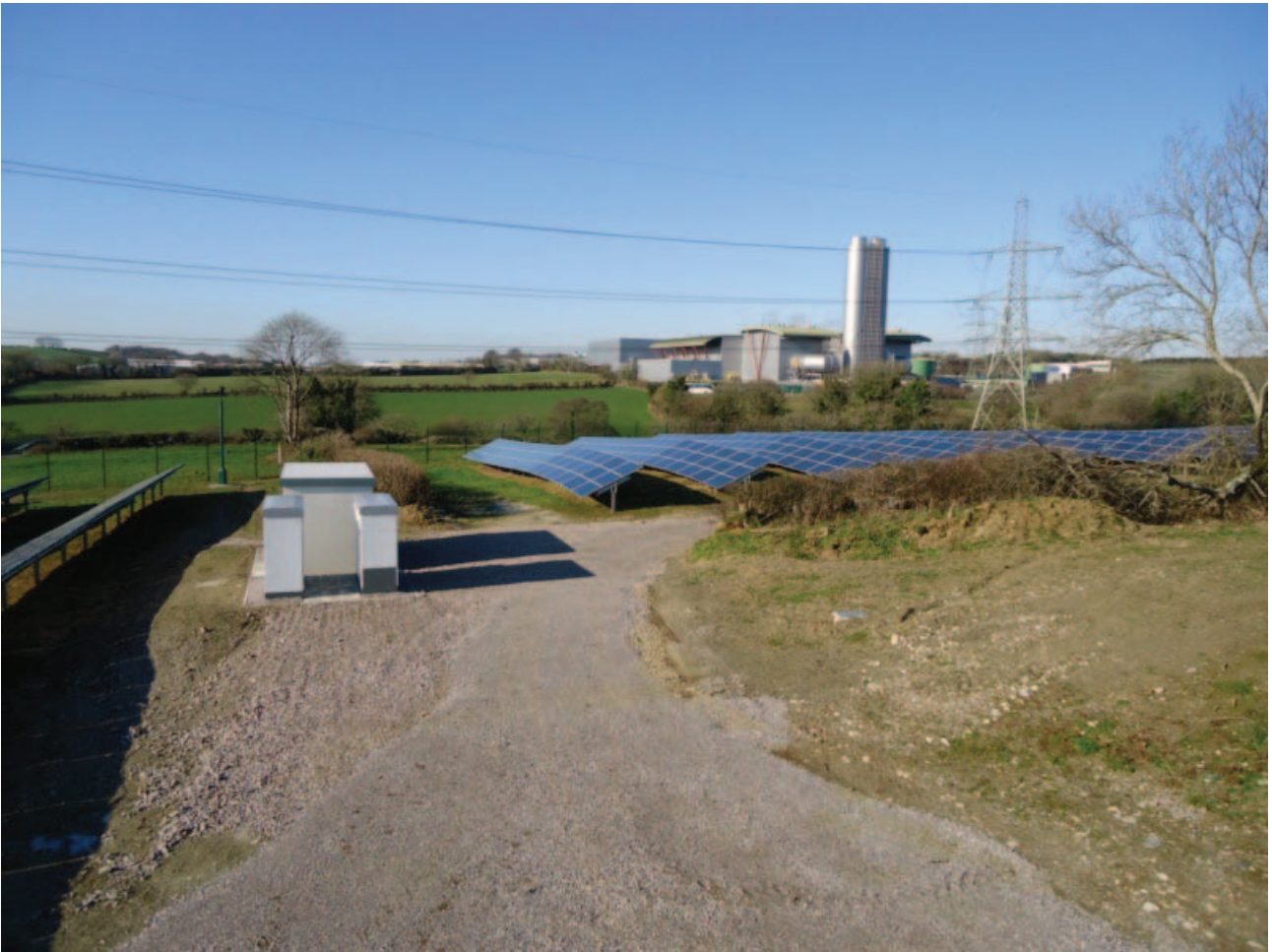
Teknikhus for inverter.
