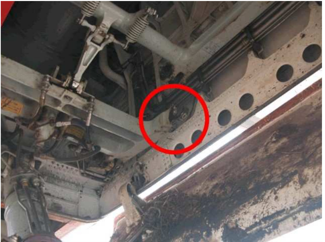
Figure 2: View of broken stabilizer brace assembly.
